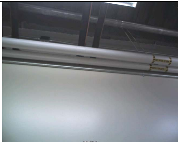
Figure 15 Air leakage around pipes penetrating the wall between the garage and the conditioned space. There are a number of locations where ducts, conduit and pipe penetrate the garage walls that must be
